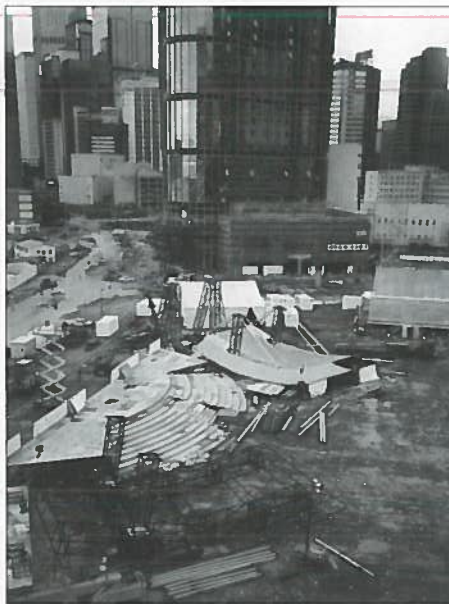
Preparations underway: above the roofs on the deck for the pre-wire and below, the first roof is lifted into position.
